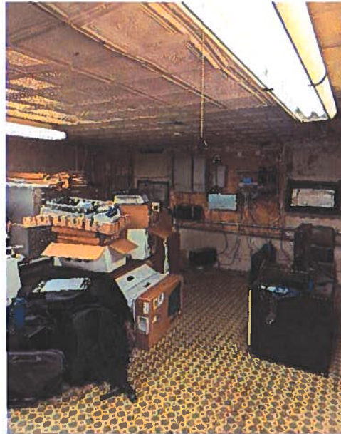
Figure 3: Existing Server Room
