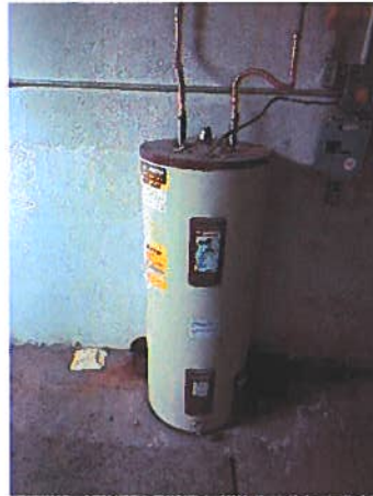
Figure 4: Existing Water Heater
