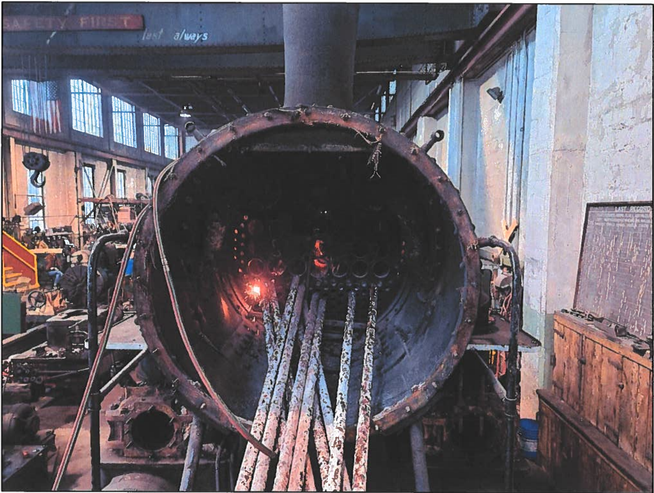
As part of the boiler inspection all of the tubes have to come out of the boiler.
